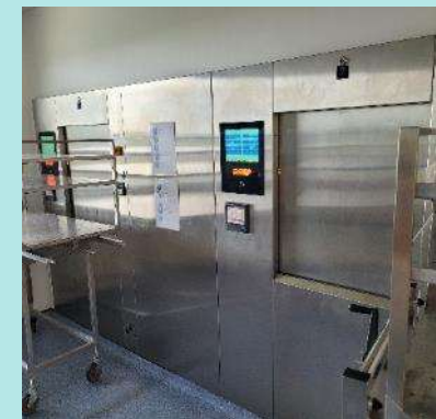
PDSE's two autoclaves at Devonport (now running 'lead and standby')
