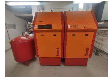
PDSE's gas boilers at Derriford (61t CO 2 e FY 23-24 - the highest emissions from boiler plant from PDSE's three directly operated sites)
